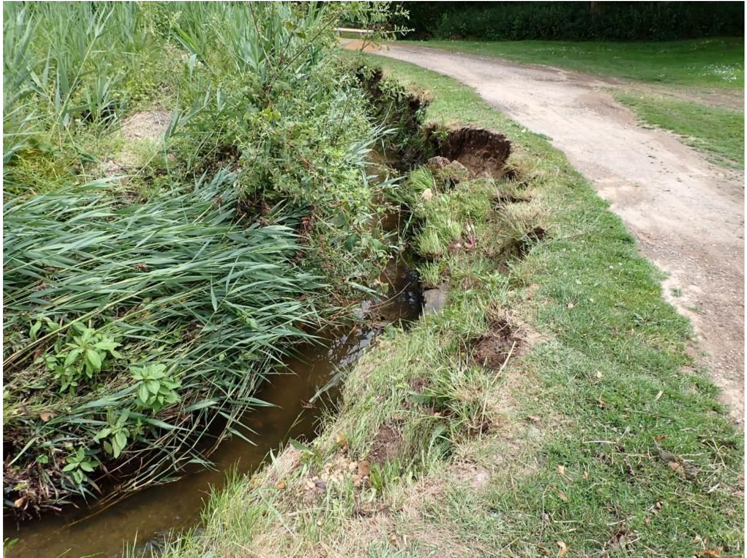
Erosion and brook bank collapse along Lye Brook lower down in the golf course area next to the south fen part of the SSSI following 20 th June 2023 rain-storm. Bridge damaged
